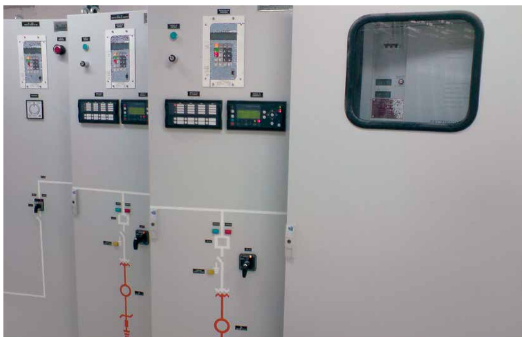
› smART P500R in cubicles.
